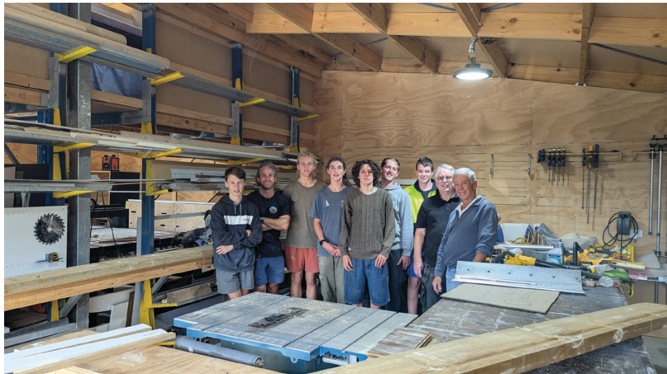
Senior students from The Village School (Royston Senior Campus) have helped construct a ga-ga ball pit Star of the Sea School in Cowes.
