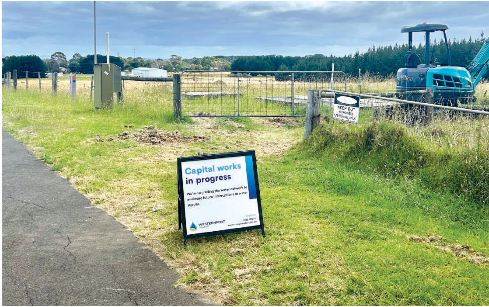
Westernport Water are upgrading the Cowes pressure reduction valve at 2102 Phillip Island Road, which will increase the flow rate of water required to meet demand for the next 40 years.
