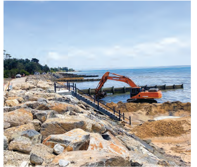
The $3.35 million, 360-metre wall in Cowes east was built as erosion defence in 2022. A new report states while sea walls may protect what is behind them, beach erosion can still occur, deflecting wave energy to adjacent properties. "The era of routine armour emplacement is coming to an end," it states.
