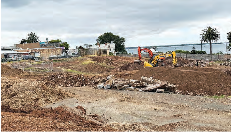
Last week dozers began pre-construction digging at 2-8 Bass Avenue and 9-10 The Esplanade, Cowes. The $130 million project is predicted to have a revised opening in mid-2026 (previously 2027).
