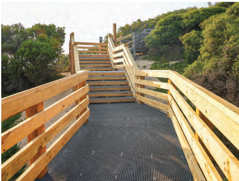
Stage 2 works include demolition of the northern stairway ahead of construction. The main beach access stairs are being upgraded after strengthening work undertaken due to erosion.
