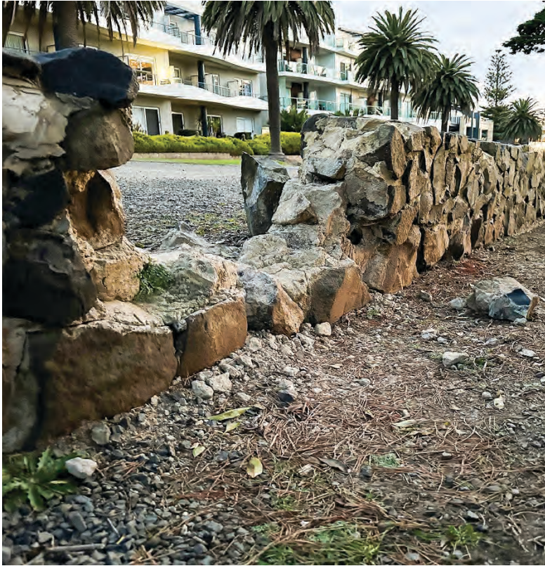
The bluestone fence at Erehwon Point continues to crumble, with no sign yet of the promised repairs for the historic wall, built in the 1950s.
