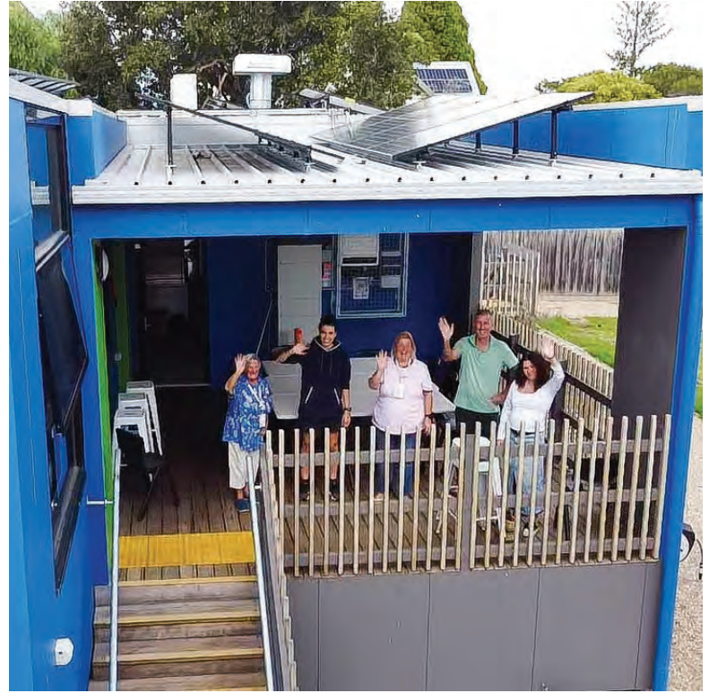
PICAL staff celebrate the installation of solar panels and a battery, which means PICAL can offer individuals a place where they can recharge their mobile phones, seek shelter or potentially get a cup of coffee while the power is out for a while.
