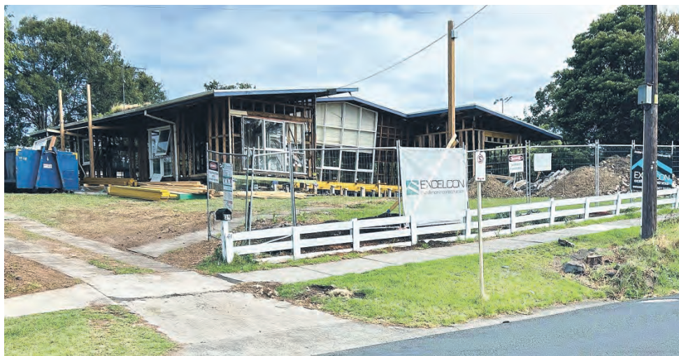
Work on a new kindergarten and long day care centre in Cowes for a 66 place facility, which has been awarded $2.2 million in State Government funding, is underway.
