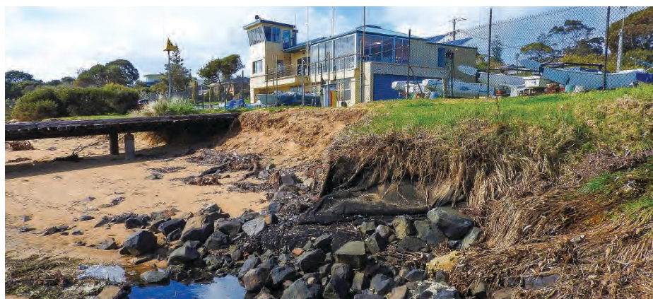
In recent years erosion has threatened to undermine the fence line.
