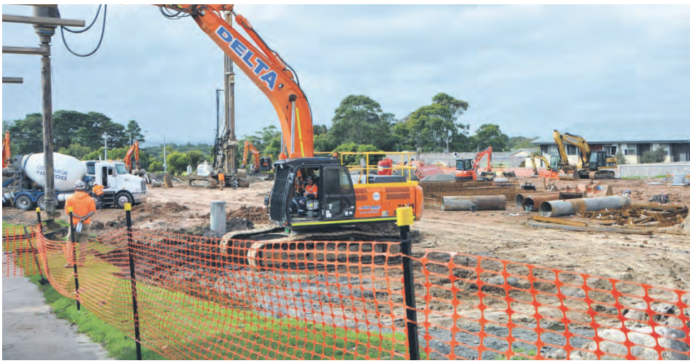
Construction is well underway on the $115 million expansion of Wonthaggi Hospital, which is due to be completed in 2023. Health Minister Martin Foley inspected the upgrade during a visit before Easter.
